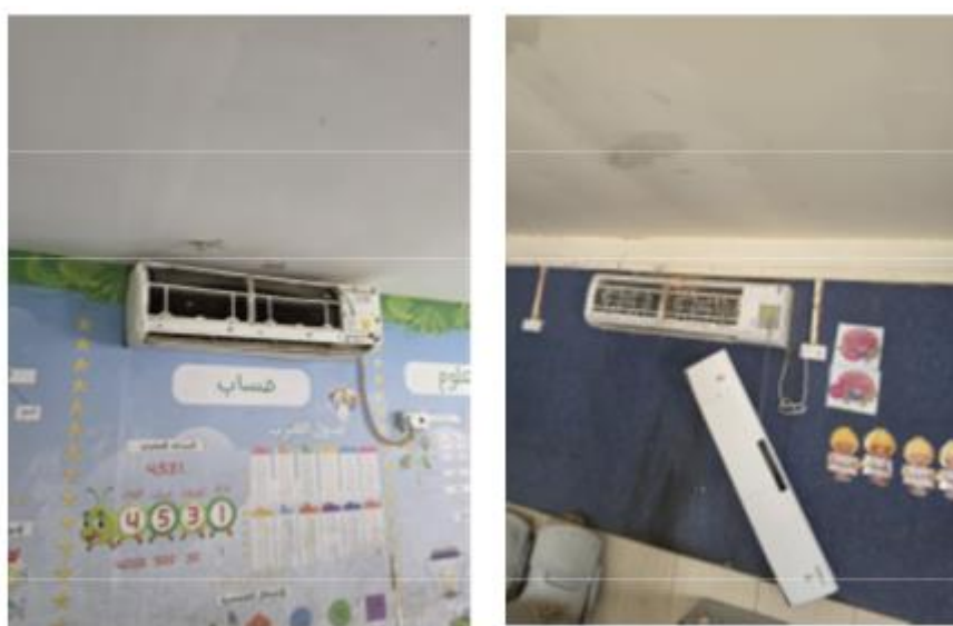
Broken air conditioners in classrooms at Al-Azazma B
