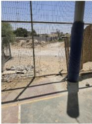
A breach in the fence at Al-Azazma B
