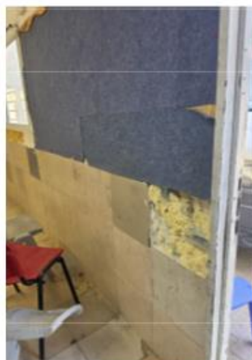
Crumbling wall cladding at Tel Arad
