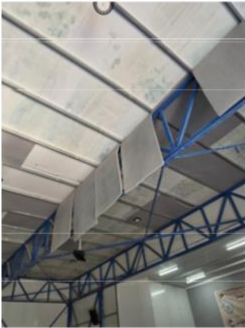
Boards and panels about to fall in the sports hall at Abu Quweider Elementary School
