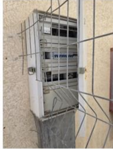
A chain-link fence adjacent to an electrical cabinet at Abu Quweider High School
