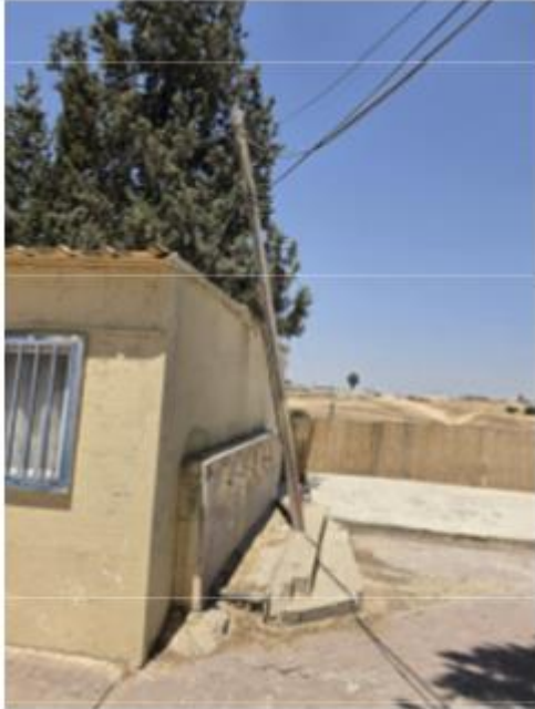
A communications pole in danger of imminent collapse at Al-Azazma A
