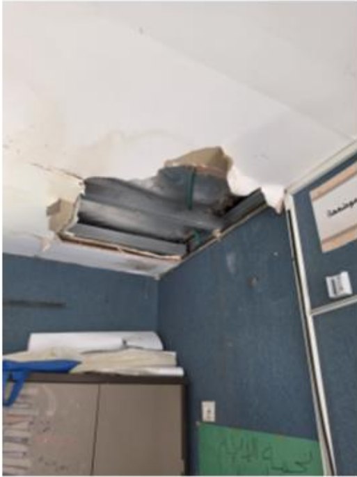
A ceiling in danger of collapse at Al-Azazma B
