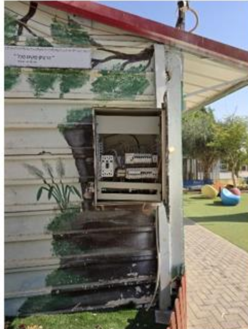
An exposed electrical cabinet, Abu Quweider Elementary School
