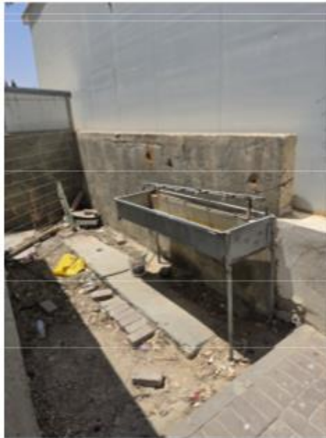
A drinking facility at the Abu Quraynat school
